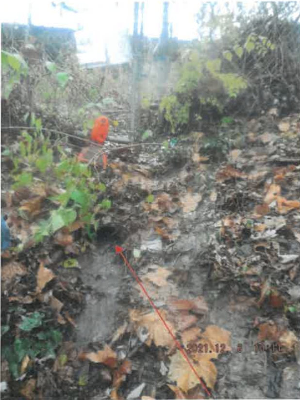
12.6.2021 – View of an unpermitted point source discharge emanating from a drop inlet in the parking lot.
