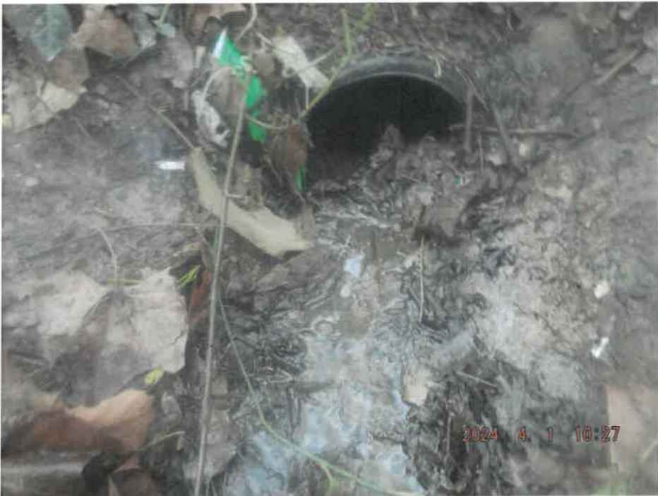
DSCF2893 - View of unpermitted outlet (previously outlet 001). Note a slight oily sheen was observed in the stormwater discharging from the pipe.
