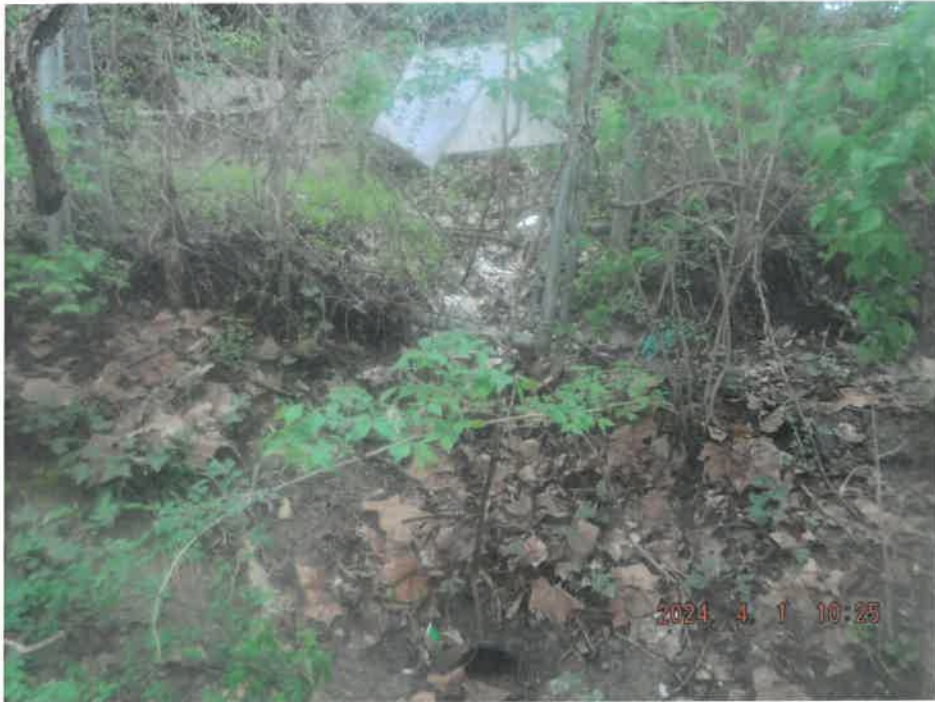
DSCF2892 - View of the unpermitted outlet which emanates from a drop inlet within the M&M Fibers facility.
