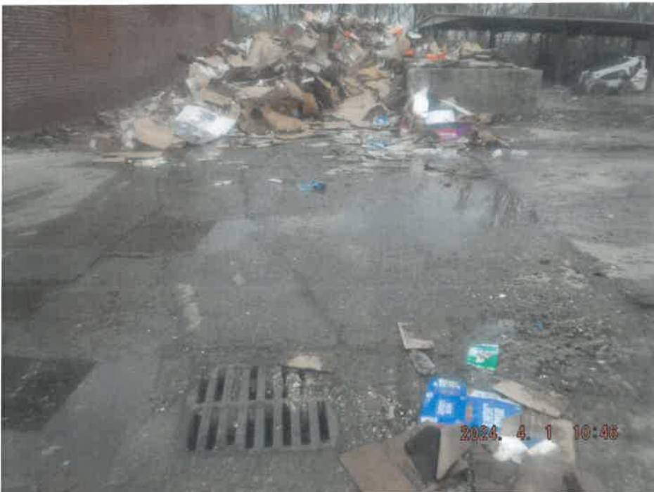
DSCF2897 - View of the drop inlet which discharges to an unpermitted outlet.
