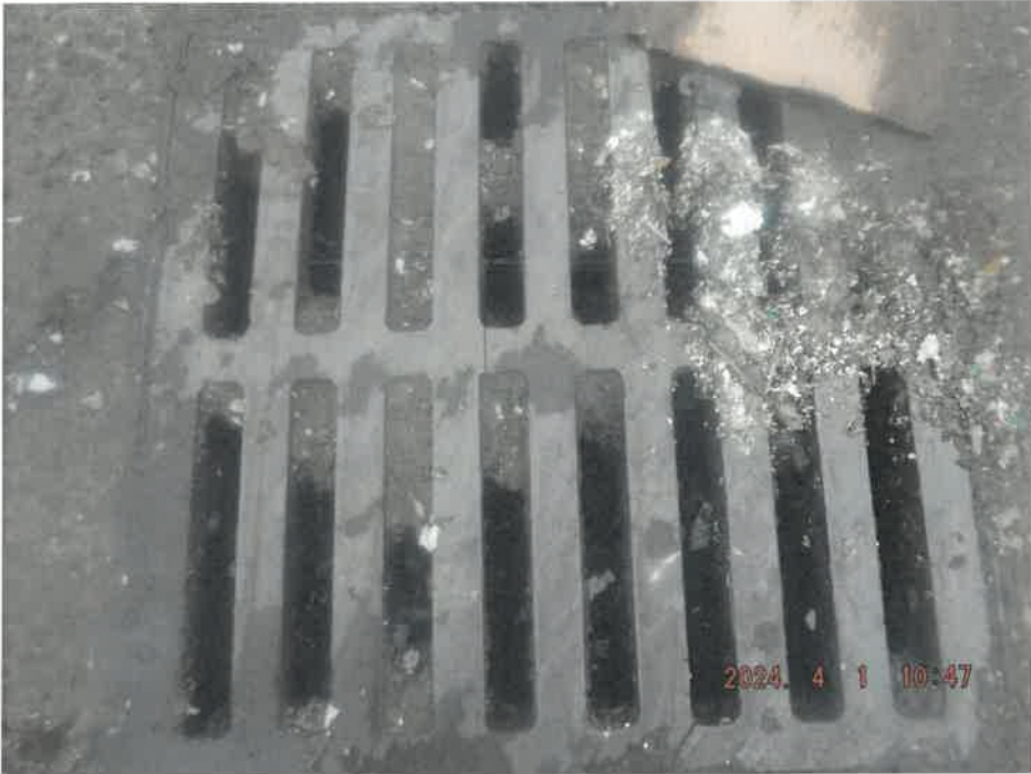
DSCF2898 - View of the drop inlet shown in image DSCF2897. Note the accumulation of solid waste on the grate and inside the drop inlet.
